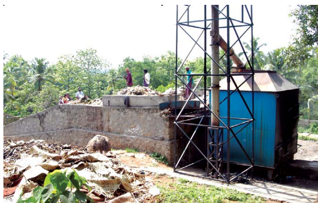
Fig. 3.4.4.1 Solid waste management system installed at Kottarakkara panchayat
