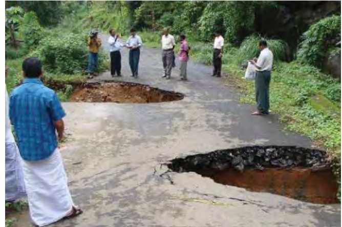
Fig. 2.1.1.2 Nilambur–Nayadumpoyil road affected by debris flow landslide at Pasukkadavu in Vadakara Taluk of Kozhikode district.
