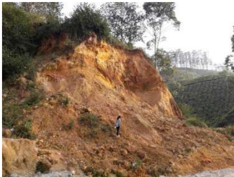
Fig. 1.6.1 A landslide along the road cut section in Munnar. Note the fallen accumulated deposit in the foreground
