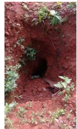
Fig. 1.6.4 Exterior view of a soil pipe. Note the loose material at the mouth of the pipe
