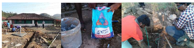
Fig. 3.4.5 Installation of Ring conductor pipes, earthing compound and connections at the four sides
